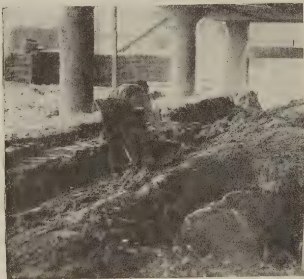
Fig. 3 shows the operator guiding the digging slip, as it is being drawn to the loading machine, shown in Fig. 4. It will be noted that this method of excavation is possible under limited head room conditions
